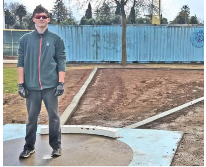
As his Eagle Scout Project Ethan Gossard installed two 6" concrete curbs around the shot put courts at Lee Middle School. In addition to Ethan's time spent planning, the project required more than 130 hours of labor from scouts and adults in our troop, plus more than $600 in supplies. The project was sponsored by the Lee Booster Club.
